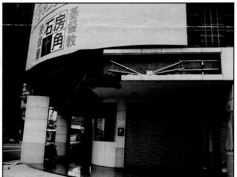
Church signs and porch destroyed by Typhoon Morrakot
